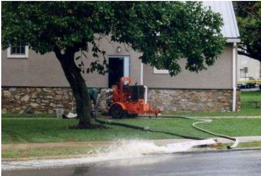
Water being pumped out of lower level of building that houses Hellertown Borough Hall and Police Station.
